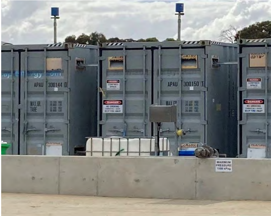
Figure 9: Fuel Storage and Fuel Forwarding Bund at BPS
