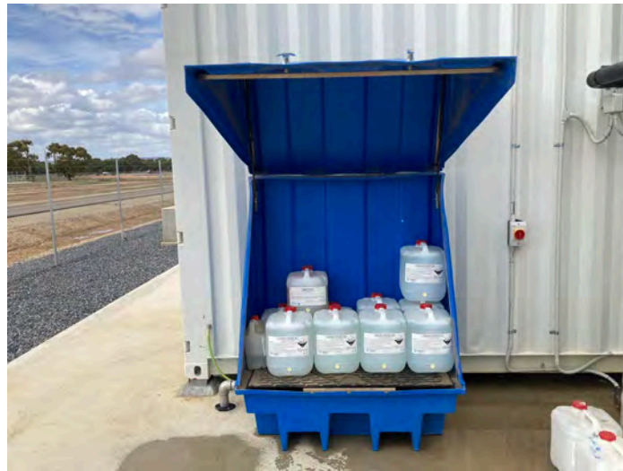
Figure 16: Chemical Storage in Mobile Bunds
