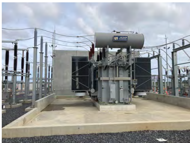
Figure 10: Main transformer at BPS
