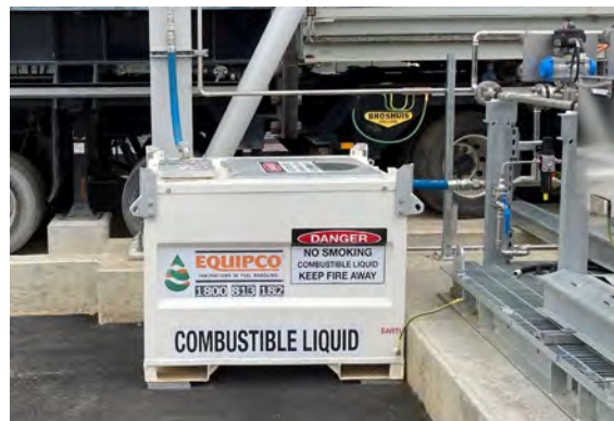
Figure 17: Turbine Fuel/Water Purge Collection Bins
