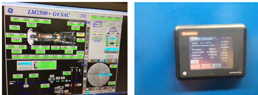
Figure 12: Control Room and RO Plant Monitoring of Demineralised Water Injection
